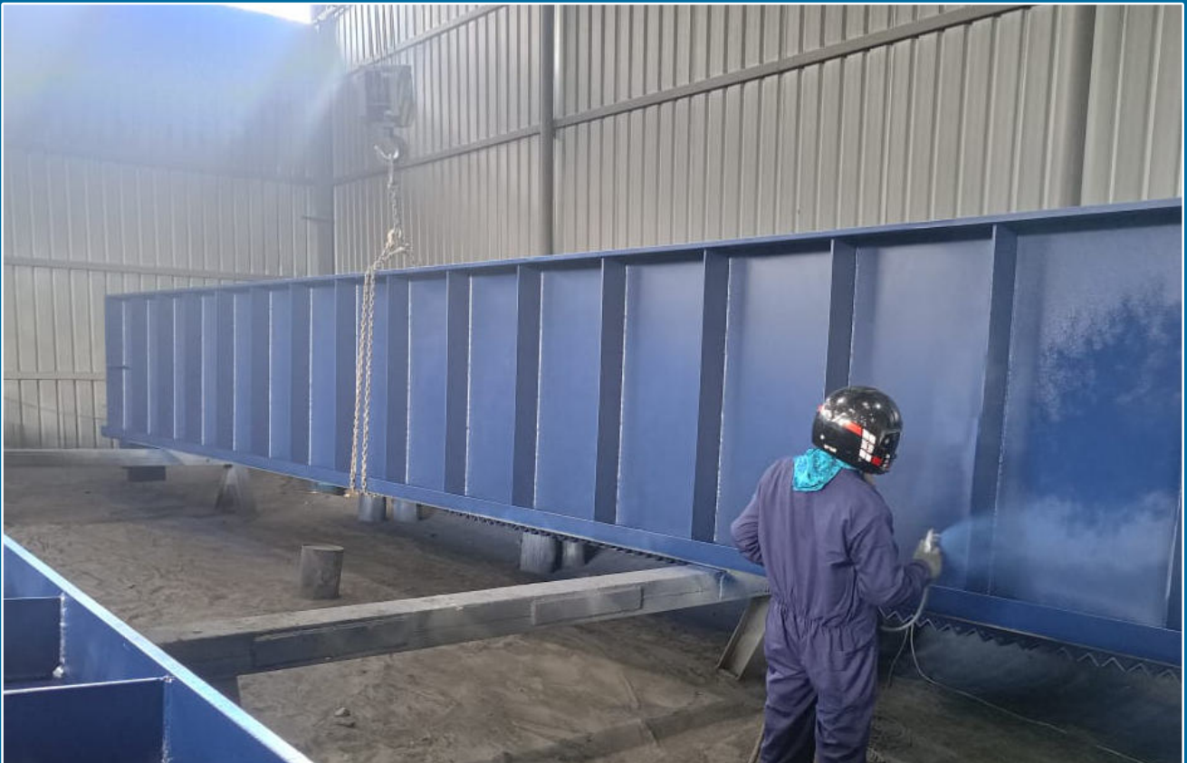
SISPL'S PAINT BOOTH
