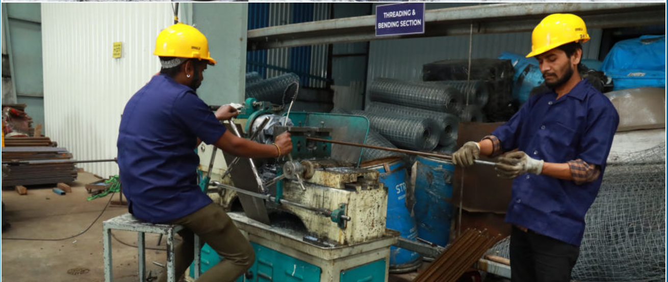
SISPL'S FOUNDATION BOLT BENDING / CUTTING / THREADING FACILITY
